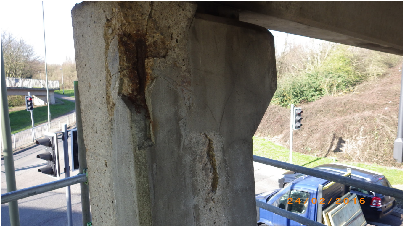
Figure three: This photograph shows the original workmanship faults of the insitu concrete material and the bearing pad in very poor condition
